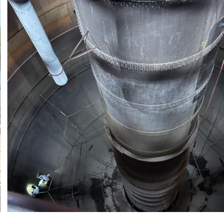
Inspection teams braved the sweltering summer heat to examine the interiors of the surge tanks—the large reservoirs in Masson. It was a rare opportunity to see them dry!
